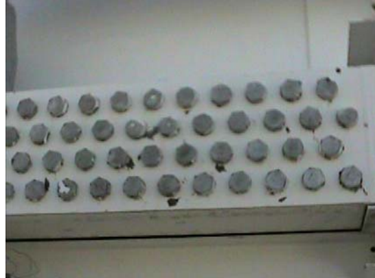
Figure 2B. Digital shot of aerial cooler header box.
