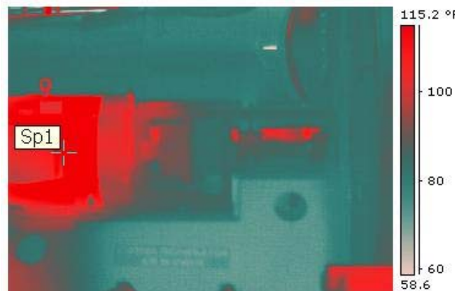
Figure 3B. Slight misalignment of coupling on incinerator blower
