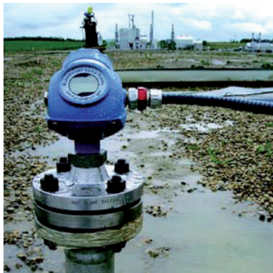
The Rosemount 5400 was mounted on a stilling well shell. The antenna was trimmed to fit the smaller pipe inside
