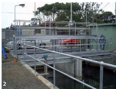
Figure 1 Two 3100 transmitters mounted on 5" diameter 316 stainless steel stilling tubes.
