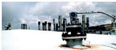
Rosemount 3300 installed on salt water disposal tank.
