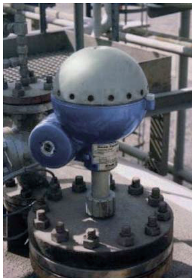
The Rosemount 5600 Radar Level transmitter is mounted on the flange on the tank roof.
