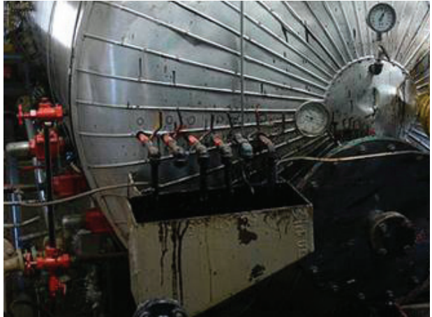
Fig 2. Bleed taps in the area near the desired interface level allow manual verification of the interface.
