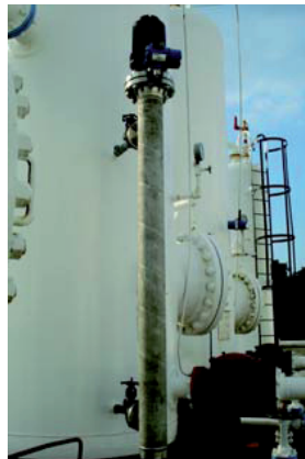
A Mobrey DS20D Level Switch with a Rosemount 702 Discrete Input Wireless Transmitter mounted on a chamber.
