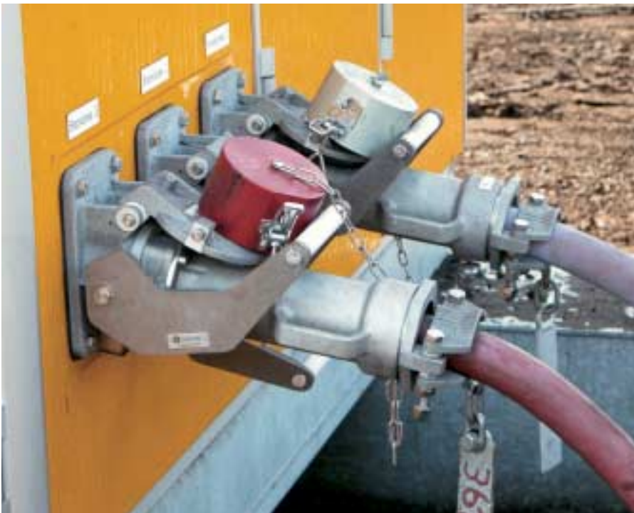
Switchgear-mounted connectors in a mine location.
