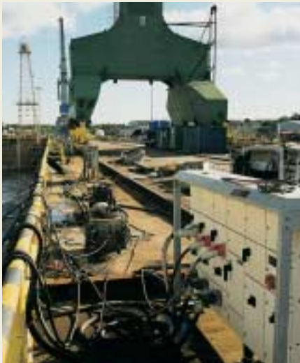
Power supply centre for a welding machine in Aker Shipyard, Finland.
