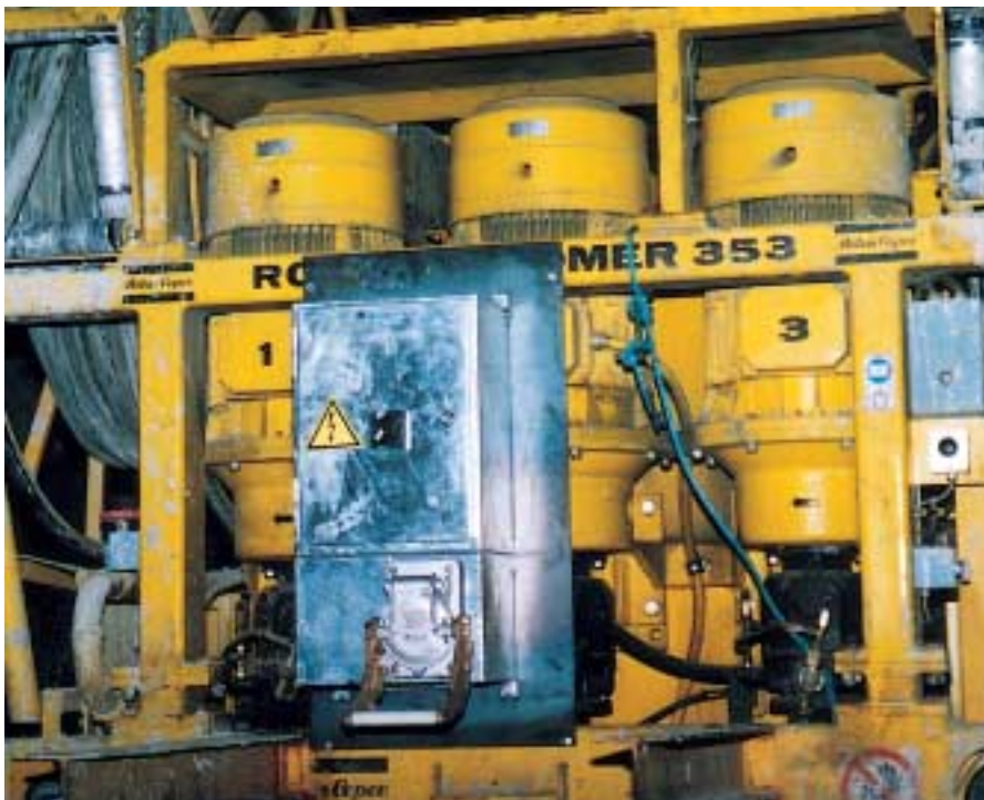
This photograph shows a Cavotec Connectors power unit used to supply power to a shotcrete machine.
