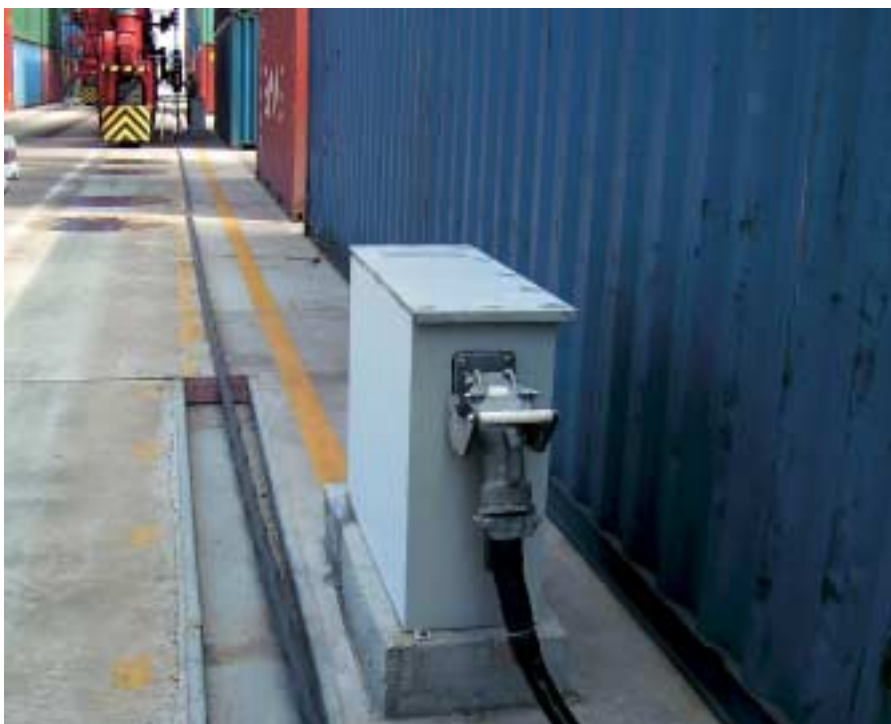
An X-type connector supplying power to a RTG (retro-fit) installation.
