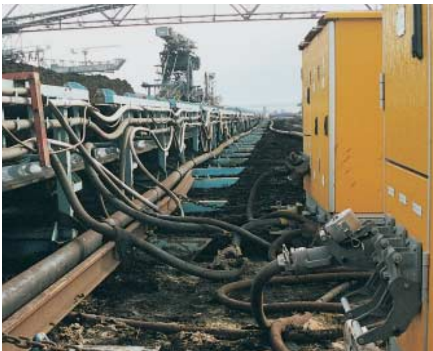
Thanks to their robust design these connectors are often used in harsh environments such as this open pit mine in Germany.
