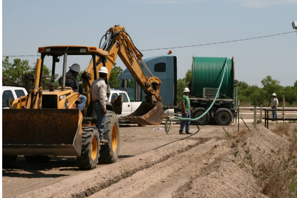
Figure 7-5 Spoolable Composite Pipe (SCP) - Unreeling Pipe for Placement in Pipeline Trench. (Photo used courtesy of Fiberspar LinePipe Canada Ltd)
