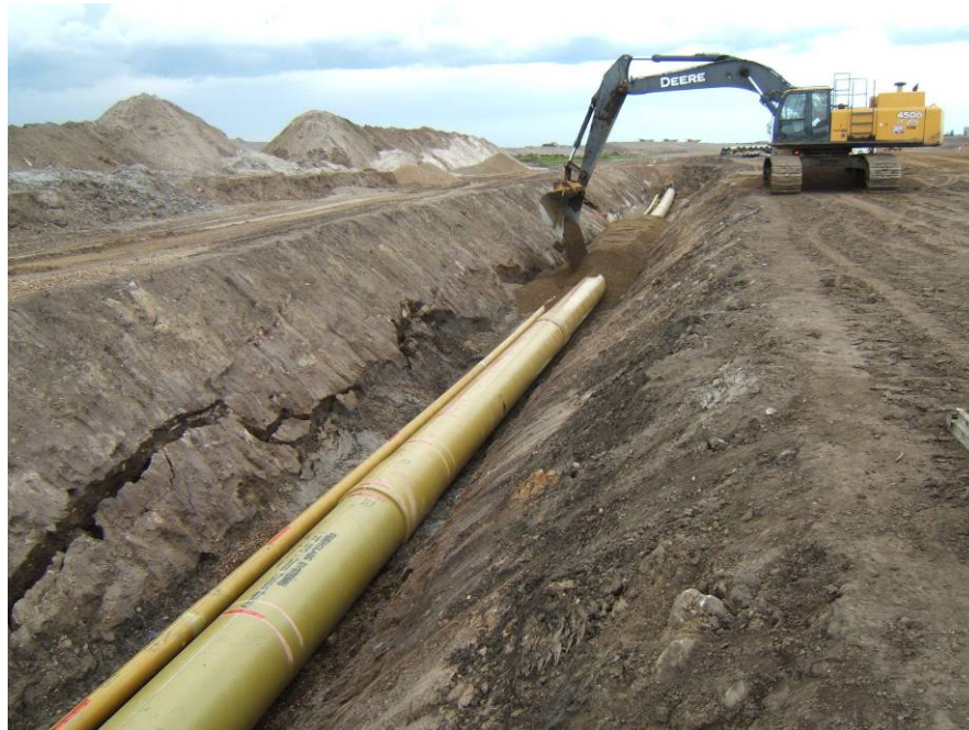
Figure 7-4 Large Diameter Rigid Composite Pipe; Placement of Select Fill Bedding. (Photograph used courtesy of Fiber Glass Systems and Fiberglass Solutions Inc)
