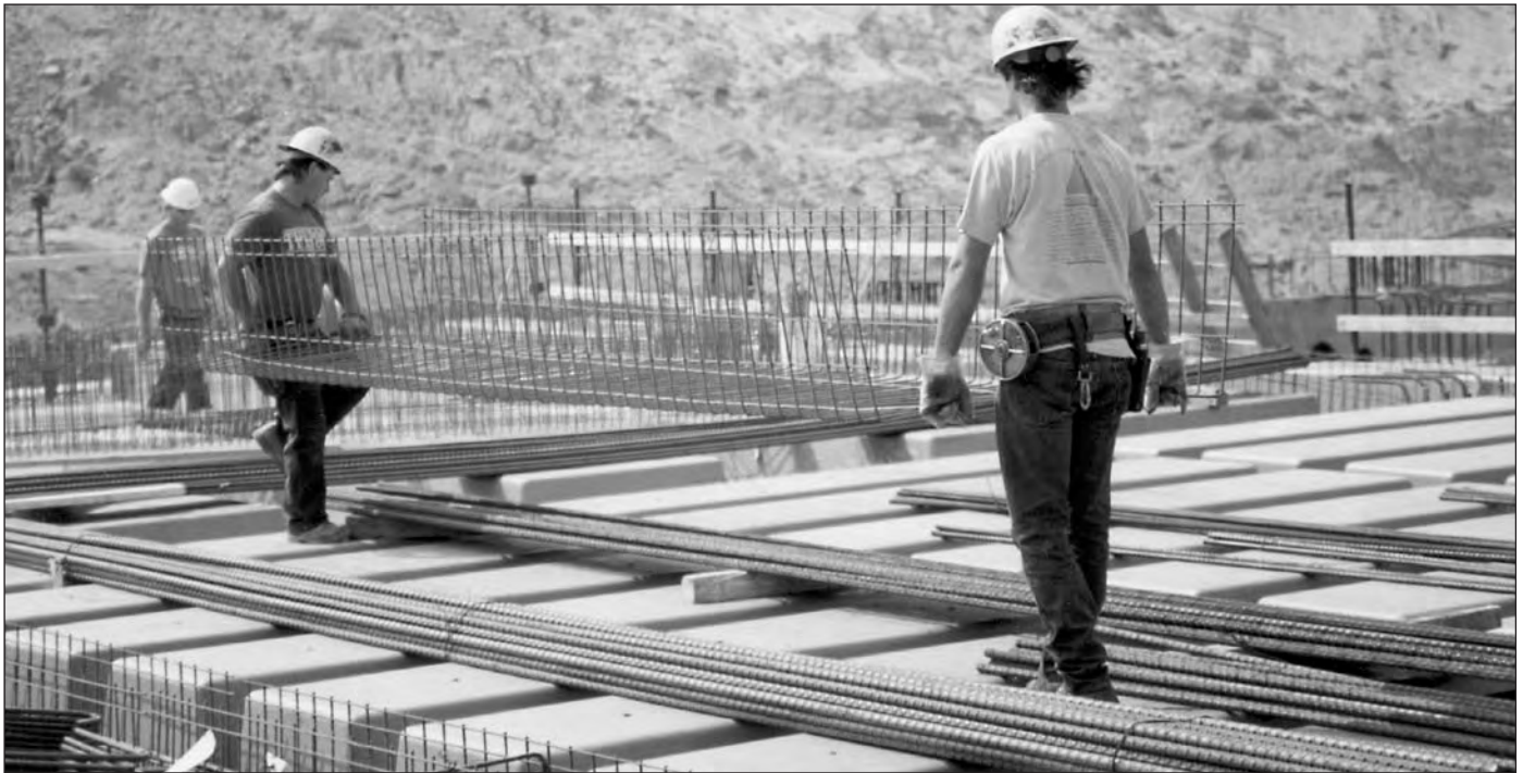
Placing a shear cage of welded wire reinforcement in a concrete girder for a sports stadium.
