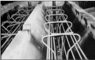
WWR used in highway median barriers.
