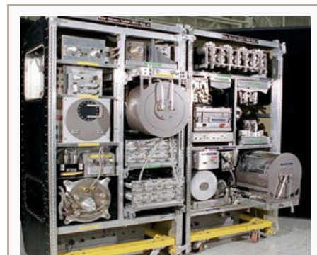
The ISS water-recycling system generates potable water after treating urine and condensate water. Photo courtesy of Flynn, NASA.
