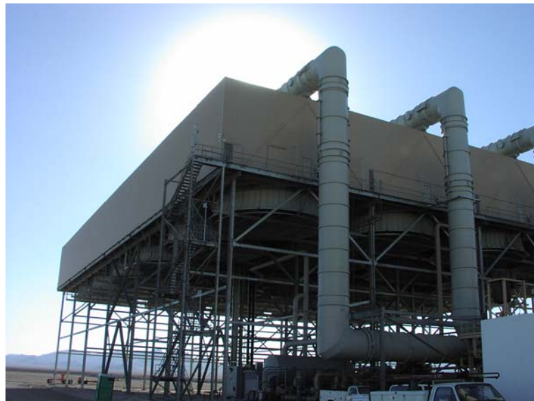
Figure 4 Air-cooled condenser showing three (of five) steam distribution ducts.
