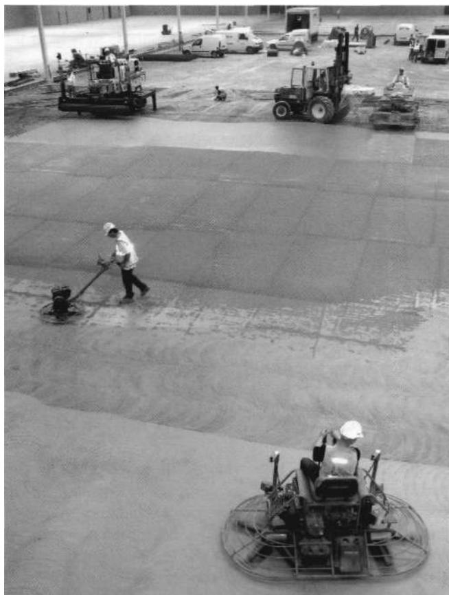
Figure 2.2: Large area construction. In the background (left) a laser screed machine is spreading and levelling the concrete. To the right a dry shake finish is being spread mechanically. In the foreground, the concrete placed several hours earlier is being finished by a power float and a ride-on power trowel.
