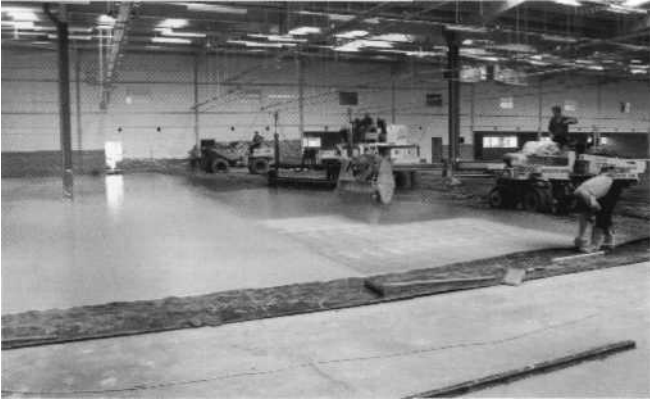
Figure 12.3: The edge of the previous pour (foreground) is protected by matting, which allows hand finishing of the edge of the new slab to be done easily and minimises the risk of splashes of wet concrete spoiling the appearance of the cast slab.
