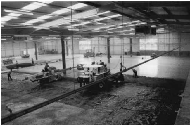
Figure 12.1: A well-laid sub-base is providing a sound platform for construction operations. Fabric is placed just ahead of the laser screed machine so it is not displaced by this mobile plant. The building is almost completely enclosed.
