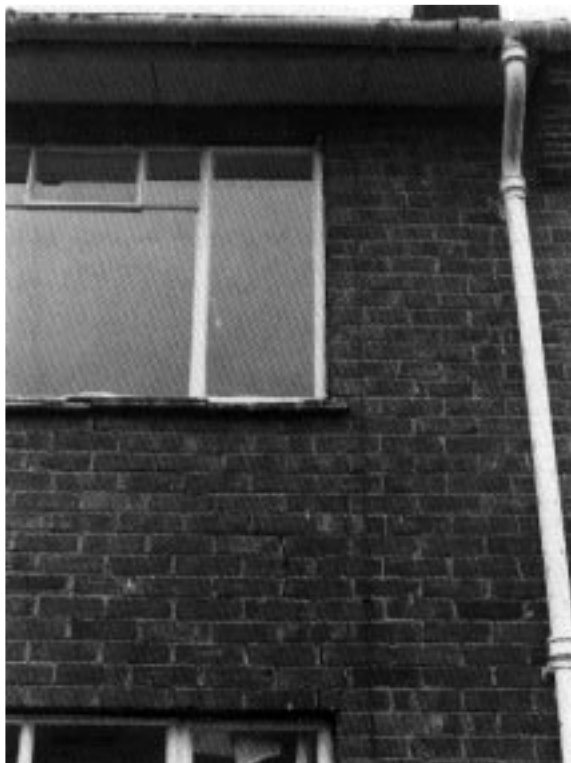
Fig 4 Category 3 damage movements predominantly rotational and horizontal
