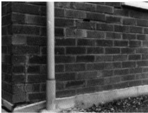
Fig 3 Category 2 subsidence damage studs are used to monitor crack width
