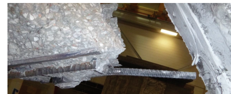
FIGURE 15: Shearing of anchor bars at the failure location.
