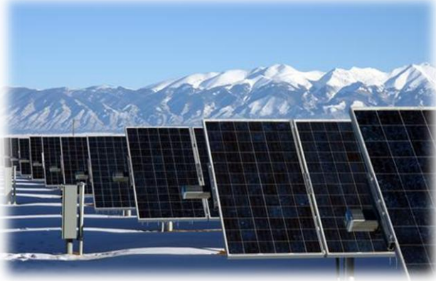
Solar Photovoltaic (PV)
