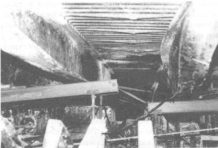
Fig. 7. Considerable thermally induced beam twisting.
