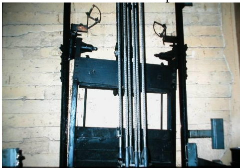
Figure 7. Derailed counterweight at 50 UN Plaza after the 1989 Loma Prieta earthquake (R Hamburger)
