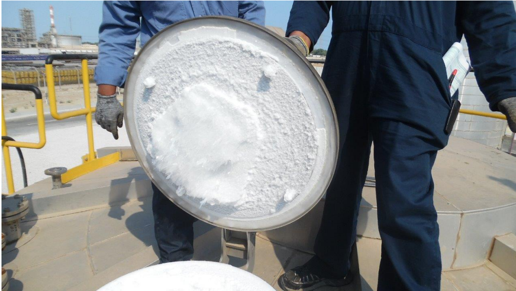
901-ERV -027 Before electrical heat tracing
