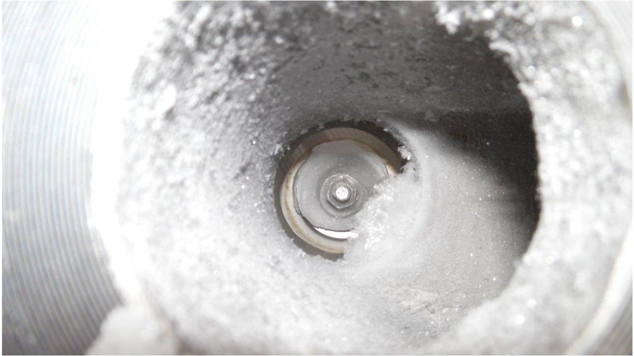
901-PVRV-027 PVRV tank nozzle fully chocec Before electrical heat tracing
