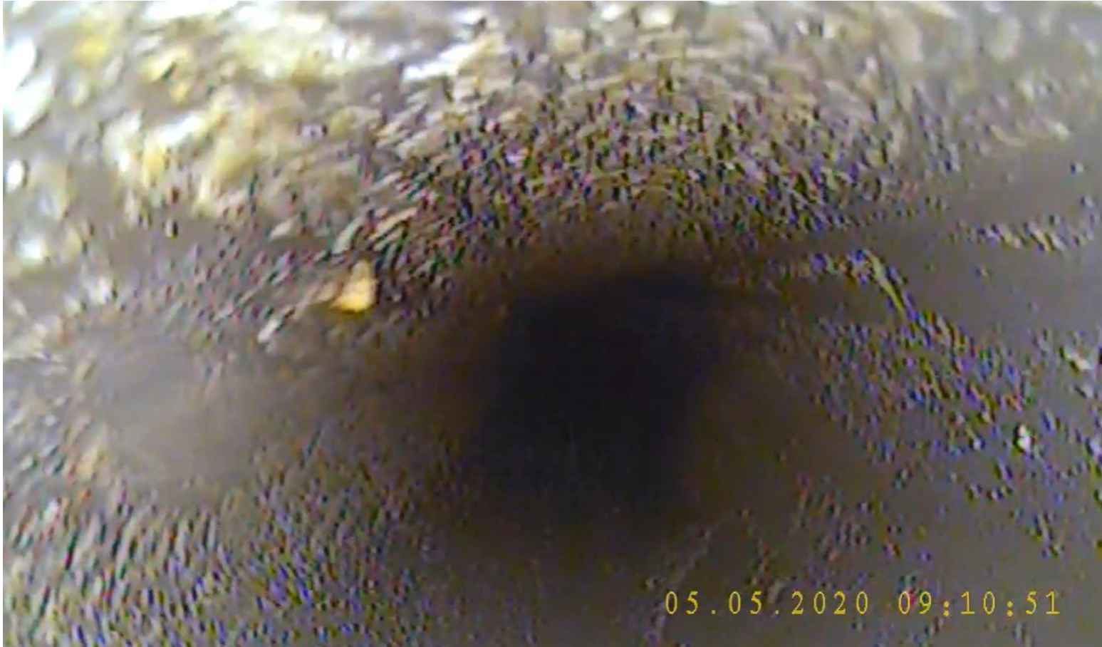
Possible evidence of pustule on pipe wall (not near a weld seam)
