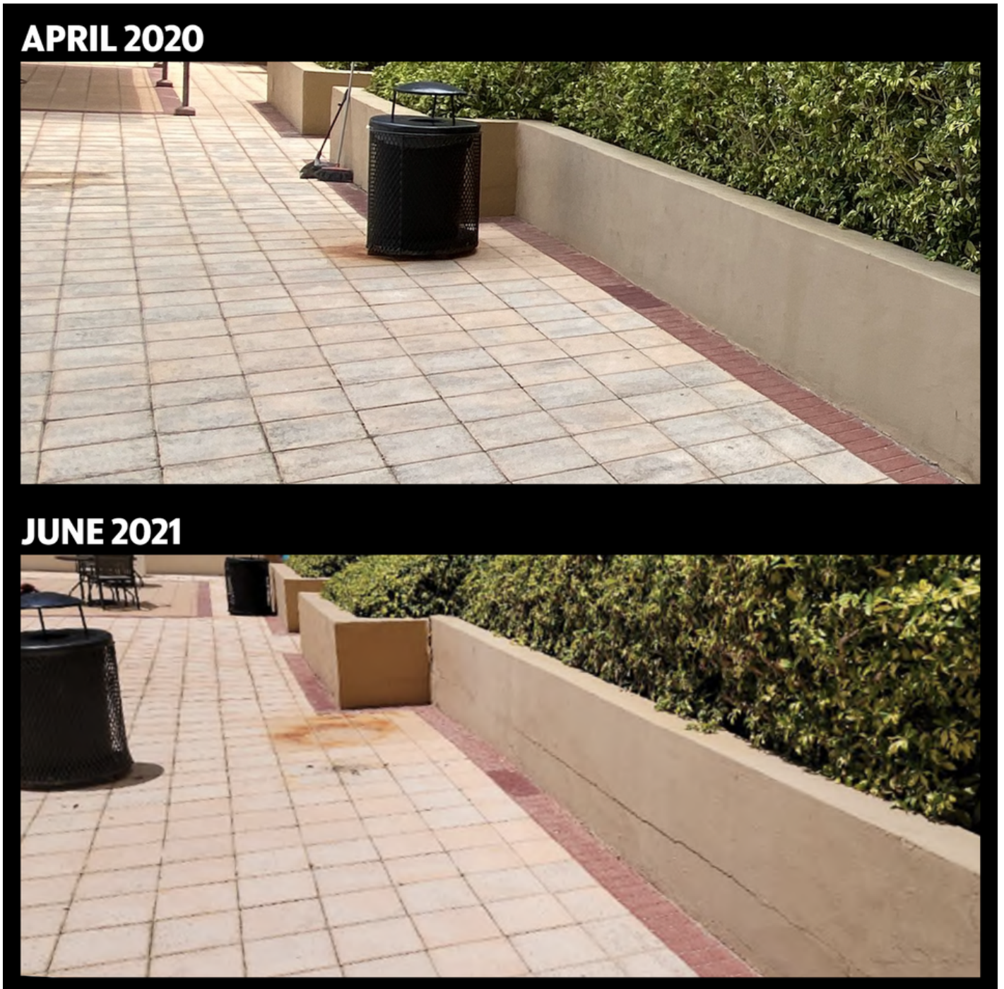
An engineer hired by Champlain South's condo association took photos of the same pool deck planter 14 months apart. The large crack that appears in the June 2021 photo was not present in the April 2020 photo. Eduardo Alvarez
