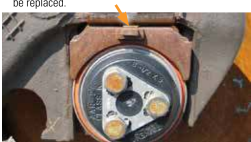
Acceptable adapter: relief is not in contact with the roof liner
