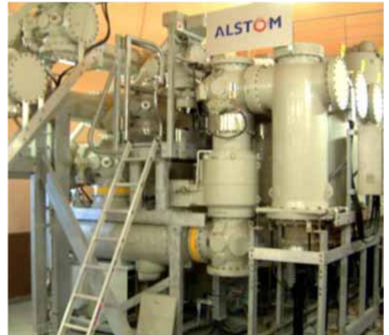
France – Paris center 245 kV underground GIS
