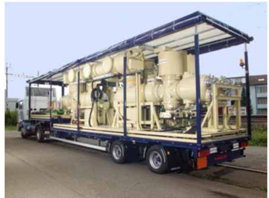
Spain – 145 mobile substation – 4 CB
