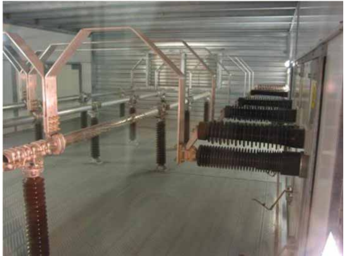
69 kV AIS in building – main busbars
