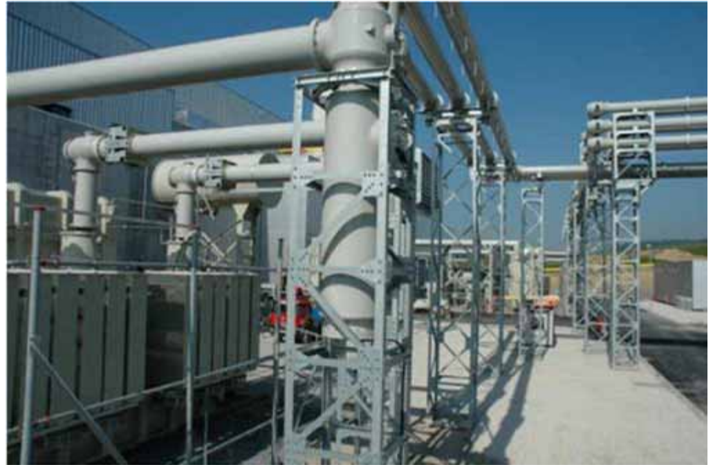
Direct transformer connection with gas-insulated surge arrester at foreground
