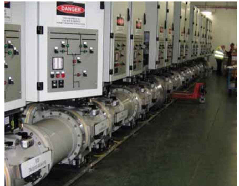
Australia – Barrow Island – 145 kV
