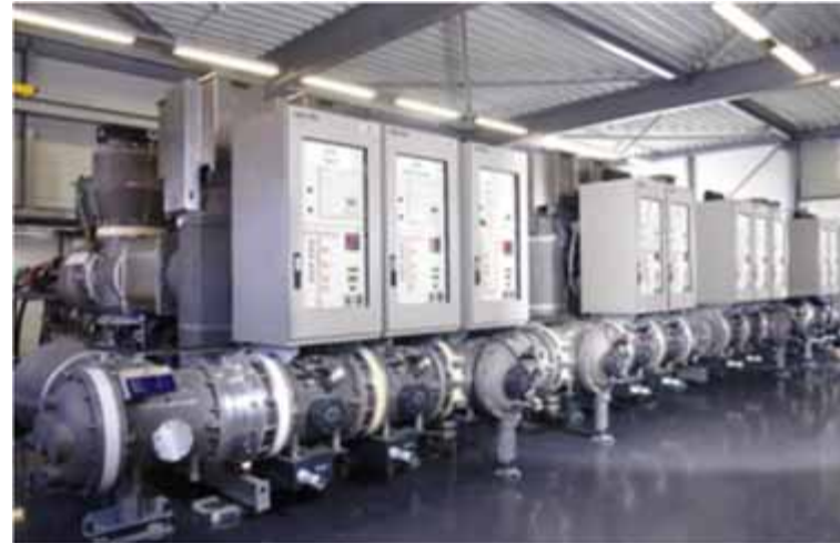
Switzerland – Wimmis - 72 kV
