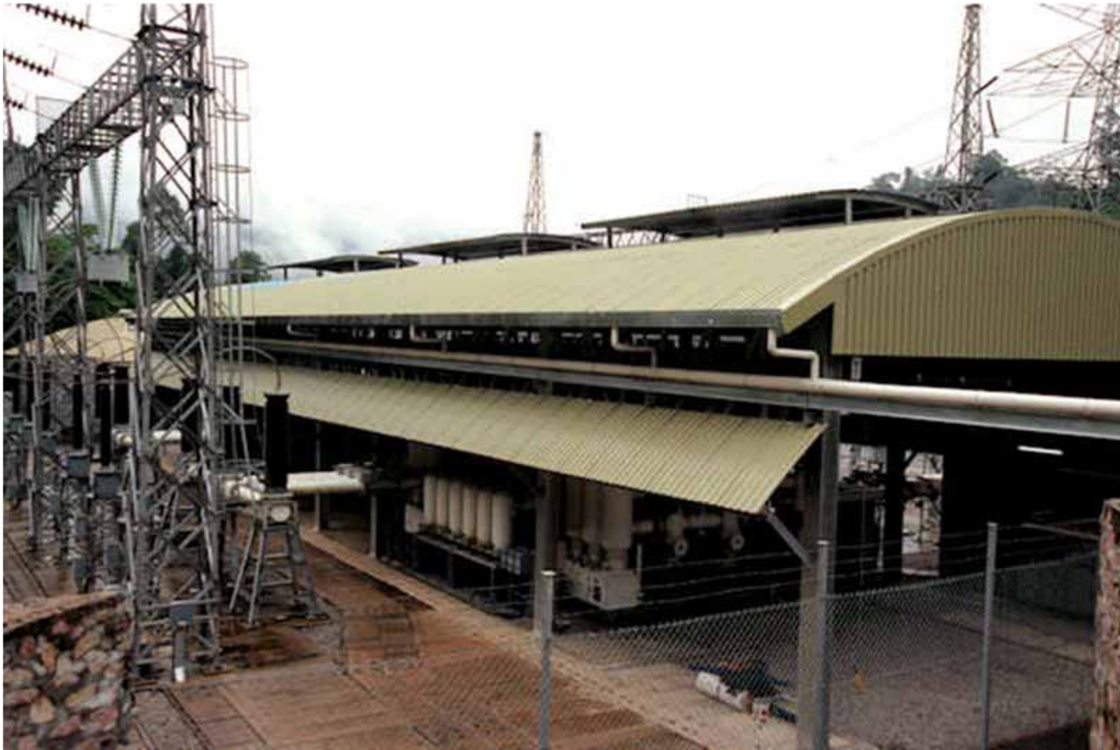
Malaysia – Pergau – 245 kV
