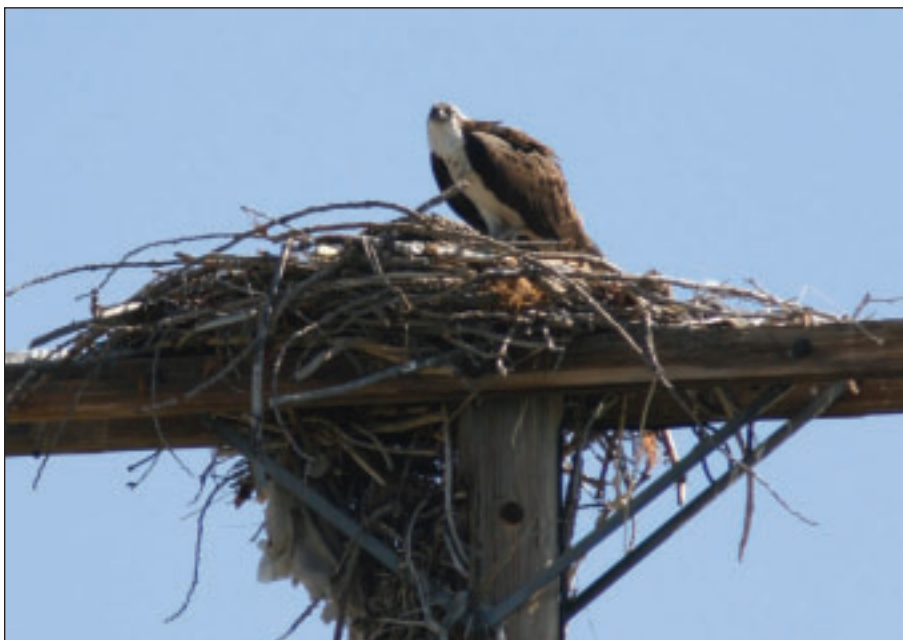
FIGURE 6.2: Osprey nest on double crossarm of non-energized pole.
