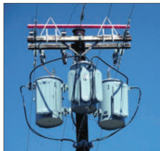
FIGURE 6.24: A pipe mounted above the conductors can be used as a nest discourager on distribution poles with insulators mounted on the crossarm. The use of triangles is cautioned against, as they may aid in the accumulation of nesting material. This design may pose an electrocution risk if exposed equipment and conductors are not covered or adequately spaced.
