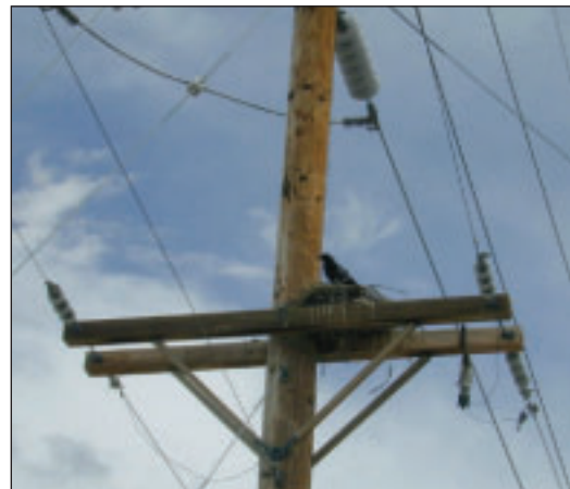
FIGURE 6.6: Common raven nest on distribution underbuild of transmission structure.
