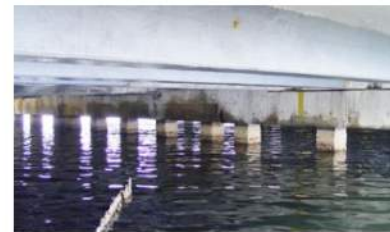
Before its replacement, this bridge developed severe corrosion.
