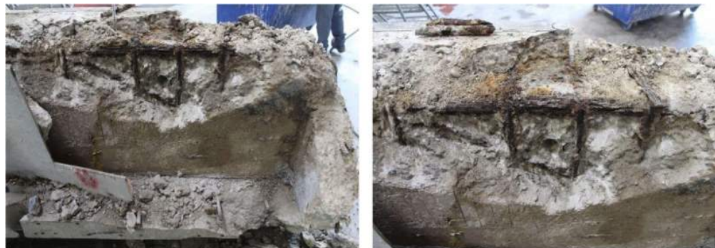
Figure 220—Corroded steel reinforcement in the north end of Girder 3-1
