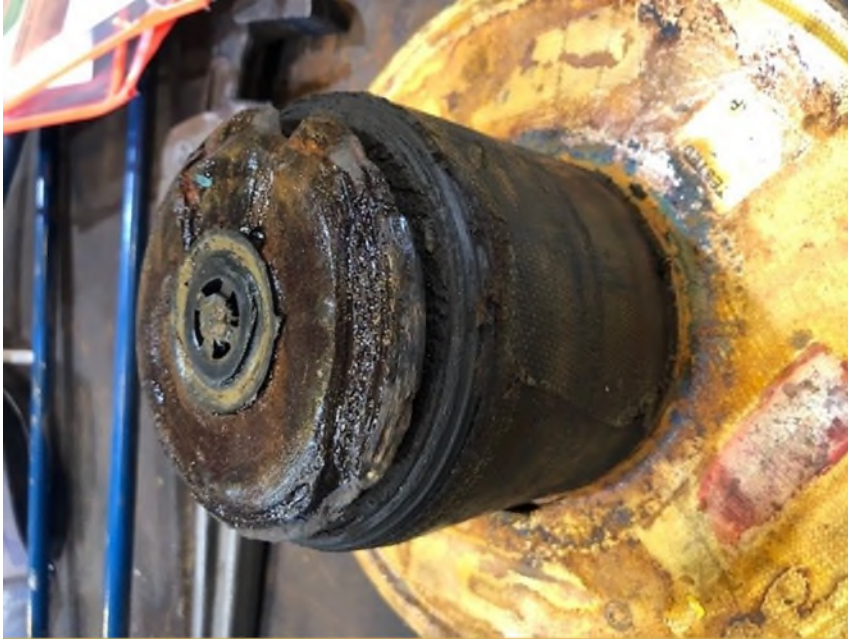
Figure 1: Containment Shell Damage
