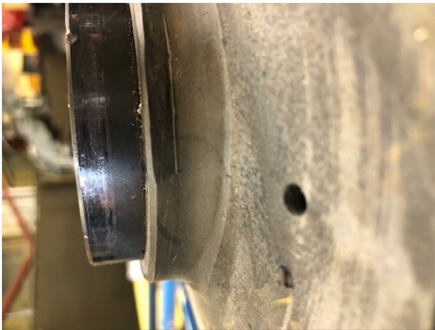
Figure 4: Impeller wear ring showing signs of dry running according to manufacturer
