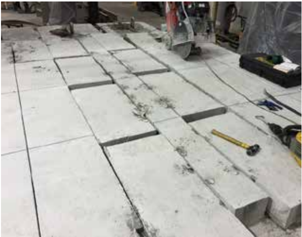
(c) Debonded Edge Pieces on Girder #2 Where Roofing Felt was Used
