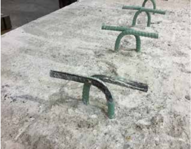
(a) Saw-Cut Damage to Rebar (Girder #3)
