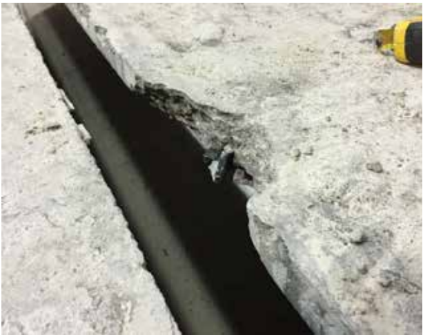
(c) Broken Flange Tip (Girder #3)
