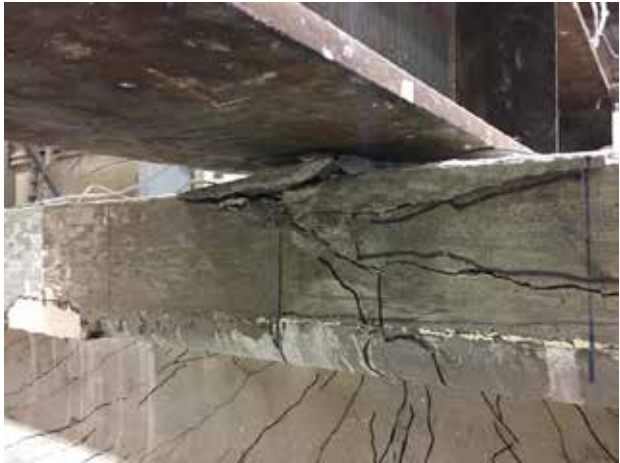
(b) Compression Zone Failure
