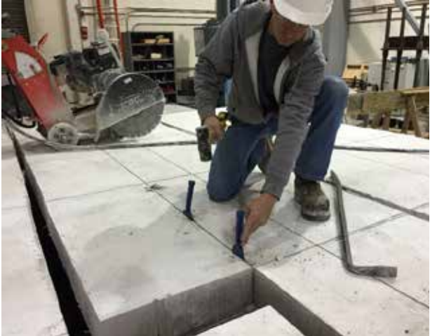
(a) Breaking the Deck Concrete Free with Hammers and Chisels Where Roofing Felt was Placed Prior to Casting
