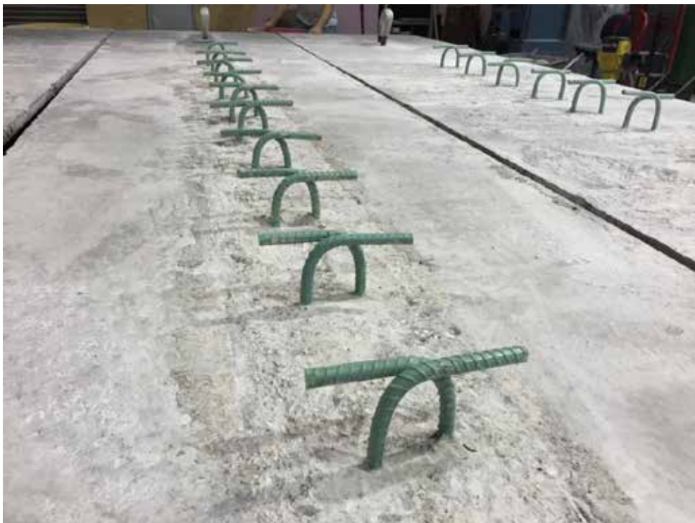
Figure 4.13: Girder #2 Surface after Deck Removal (Originally Partially Roughened with Roofing Felt over the Flange Tips)
