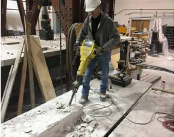
(a) Limited use of 65-lb Jackhammer to Remove Concrete above the Interface Shear Reinforcement
