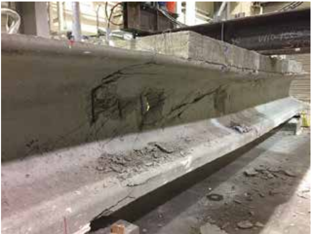
(c) Specimen after Failure
