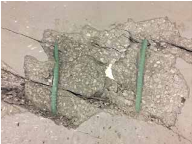
(e) Girder Web after Failure
