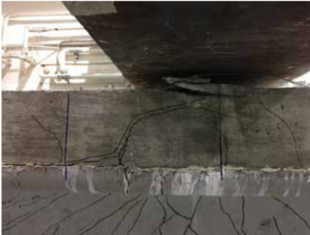
(b) Compression Zone Failure
