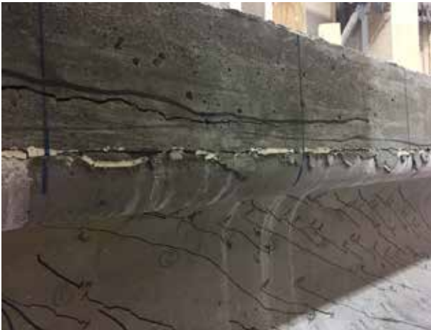
(c) Horizontal Crack Through Deck After Failure (West Side)
