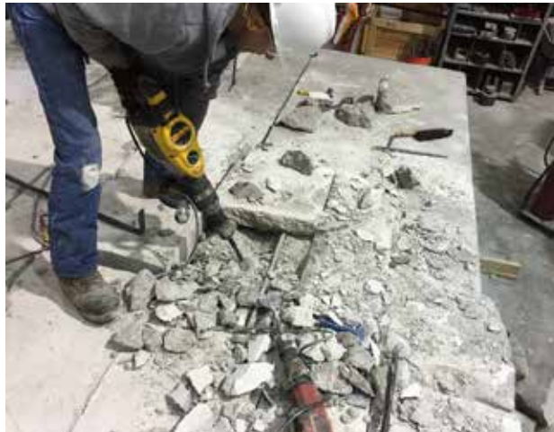
(d) Demolishing Edge Sections of the Deck Where They were Bonded to the Girder
