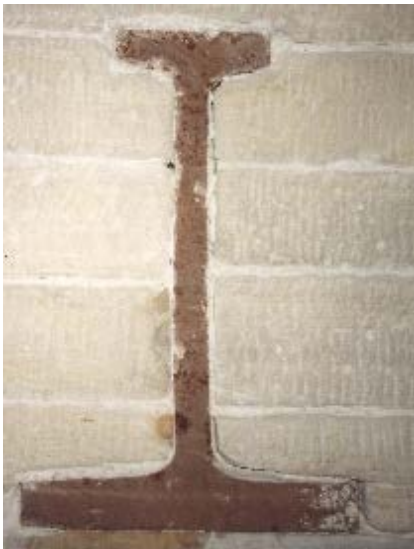
Fig. 1 End view of cast iron beam: note bubbles in cast iron, variations in flange thickness
