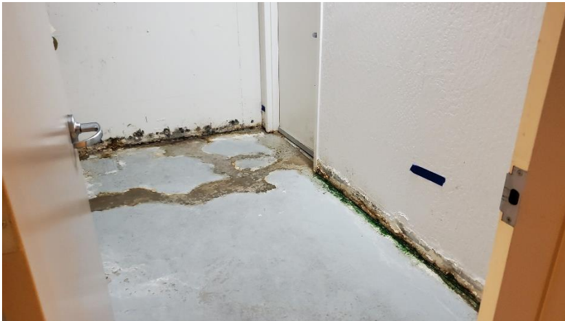
Photo 4 Signs of prior leakage in the podium at level B5
