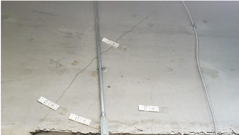
Photo 19 Preexisting cracks in tower column H-11 at B1
