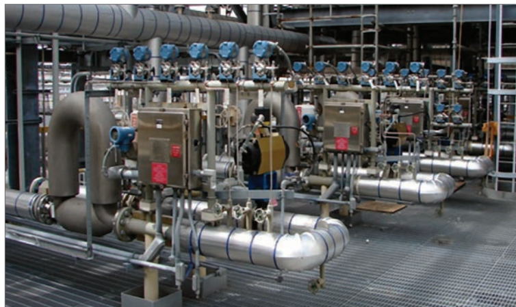
Figure 11: Hydrogen / natural gas blending system.
