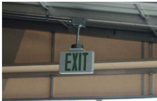
Figure 5. When public decks have an occupant load of more than 50 and serve as a means of egress, illuminated exit signs may be required.
