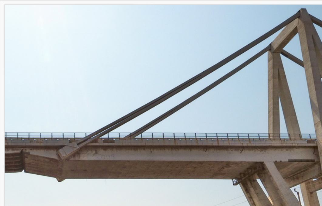
Pylon 9: The cable stay consists of two distinct stays in their lower part which merge half way up towards the tower (Hasen 2015)
